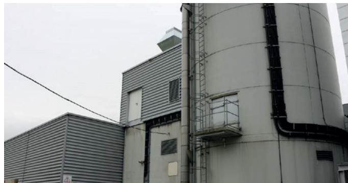
Moser built a new utility room for the new compressors (in the centre, above). The units were lowered in through the roof for installation.
