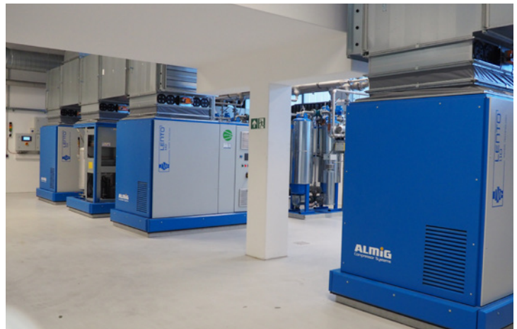
Guaranteed not off the shelf: ALMiG’s compressed air station meets very special requirements for clean compressed air.
