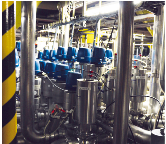
Valve terminals in the brewery are also controlled with compressed air.
