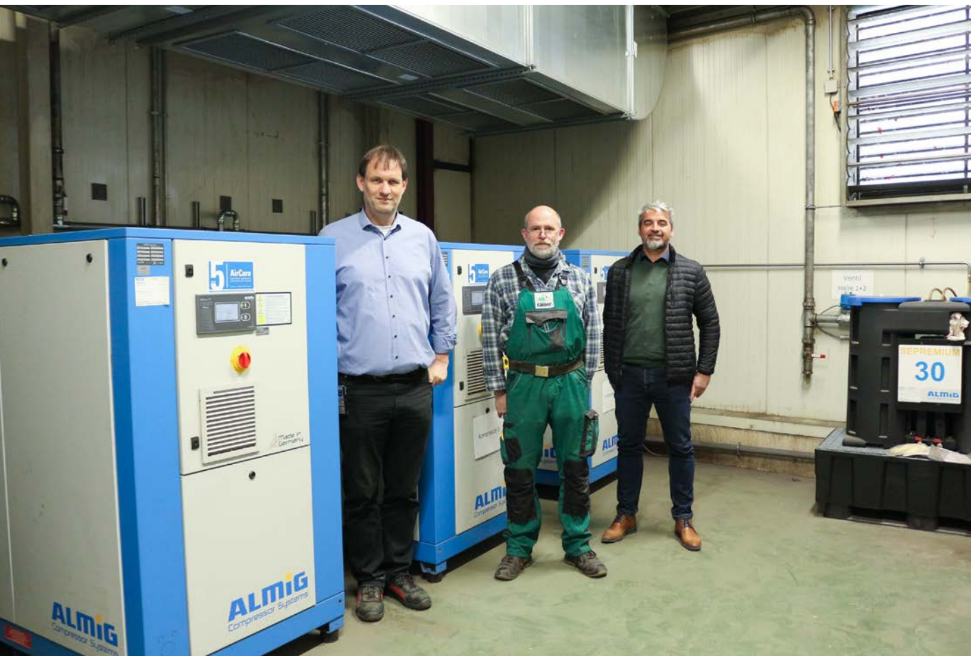
Elmar Raiser (left), Ralf Entenmann, the person responsible for compressed air (centre), and ALMiG area sales manager Michael Ziegler in the new compressor room.
