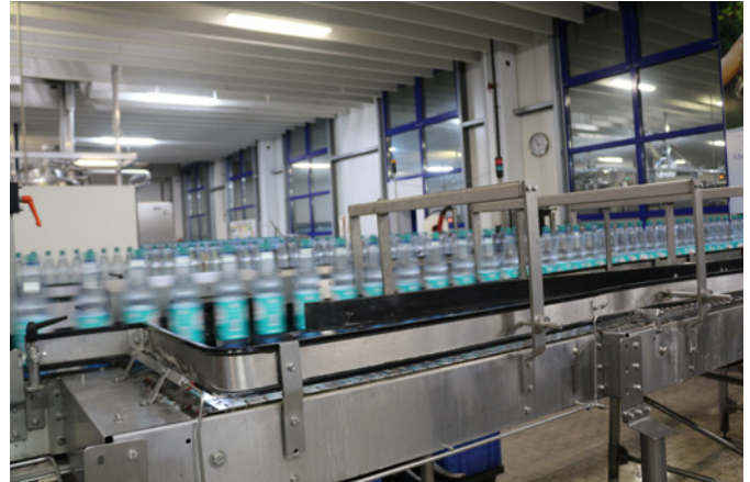
Compressed air is used throughout the plant. It is used as operating power and as control air for valves and cylinders.
