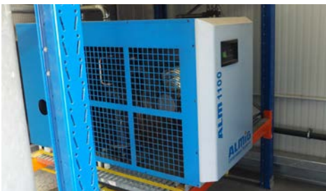
The external, refrigerant dryer: Its characteristics are precisely adapted to the respective system.
