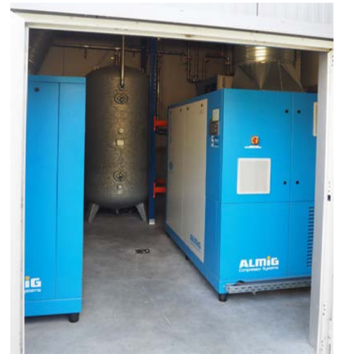
With the new compressed air tank, a volume of 3,000 liters is now available.
